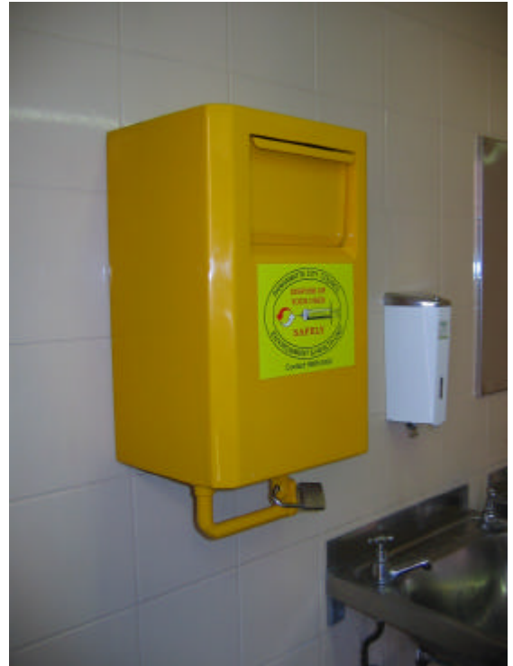
10 litre sharps bin installed within Public Toilet, Parramatta Mall.
